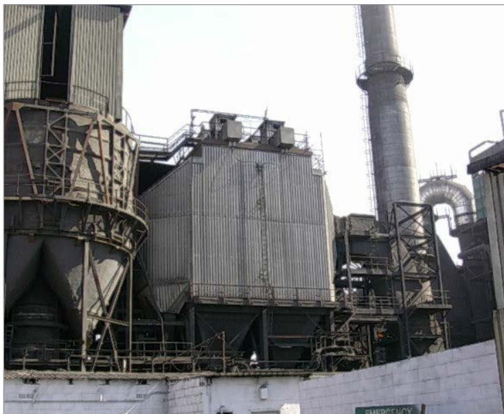
Dust Extraction Plant
