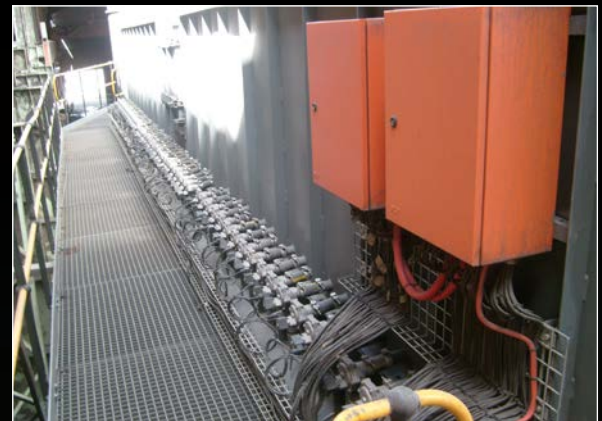
Bag filter air pipes
