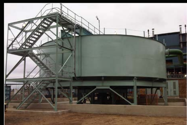
15m Ø Clarifier in operation
