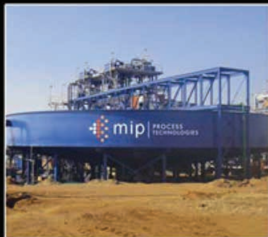
26m \phi Thickener in operation
