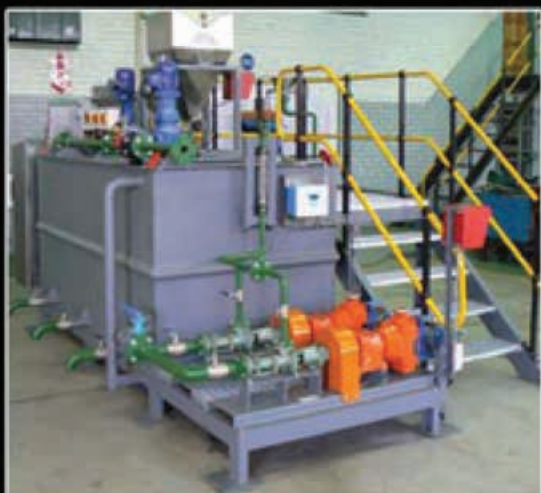
MIP-200 Flocculant Plant
