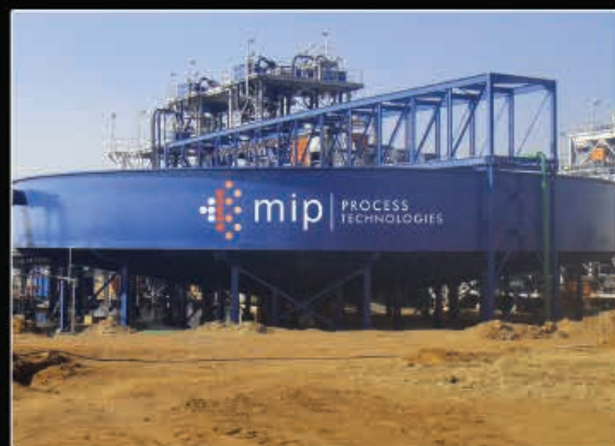
26m \phi Thickener in operation
