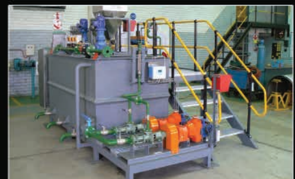
Skid mounted flocculant plant
