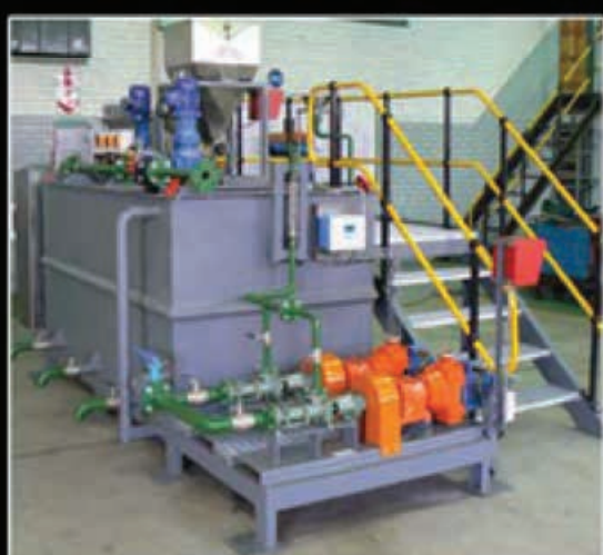
MIP-200 Flocculant Plant
