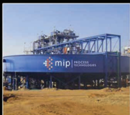
26mφ Thickener in operation
